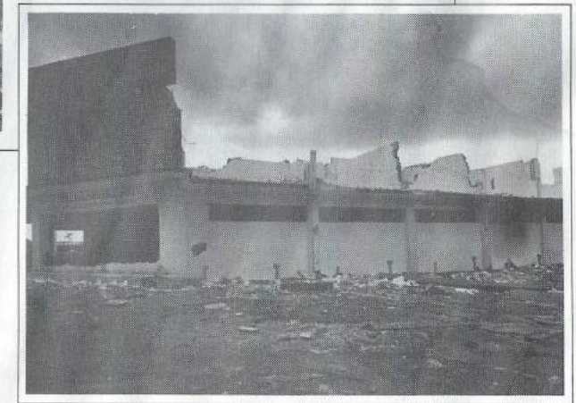
Destroyed civilian and military installations.
