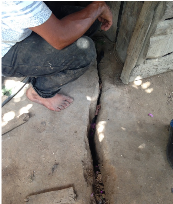
Fissures under La Cuchilla homes, due to extensive use of explosives underground, by Pan American Silver. Photo: UNBC/Rights Action field school program, 2016.
