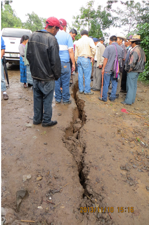
Large fissures have regularly opened in throughout San Miguel Ixtahuacan and Sipakapa, due to use of explosives in over 150kilometers of tunnels.
