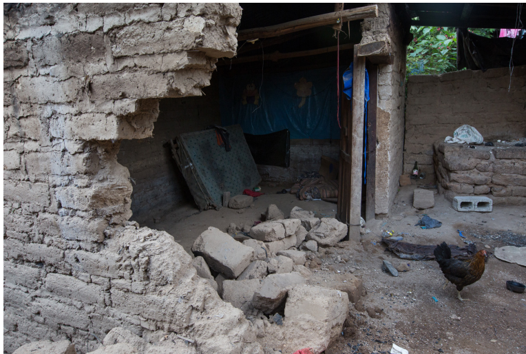
(An abandoned home in La Cuchilla , that crumbled and partially caved in due to tremors caused by the use of explosives in Tahoe's tunnels. San Rafael Las Flores municipality, Guatemala. Photo, May 22, 2016, by James Rodriguez, www.mimundo.org )
