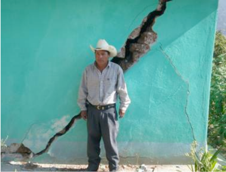
(December 2008. Structural cracks to a home in village of Salitre, due to explosives used at "Marlin" mine. Photo @ Grahame Russell, 2008)
